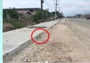
Re-enforced Concrete Lined Drains with adequate drain holes (Residence and Street sides).
